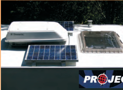
1 x 80W Solar Panel and Regulator Fully Installed
