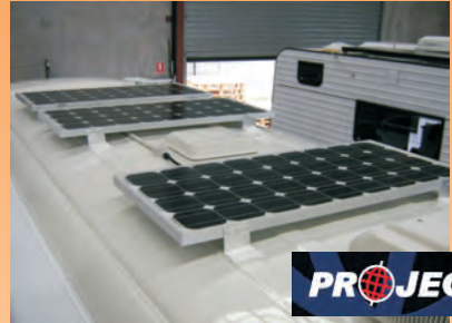
1 x 120W Solar Panel and Regulator Fully Installed
